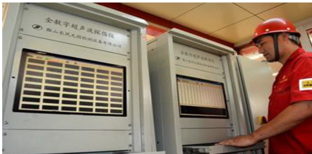
Continuous Monitoring Equipment of Ultrasonic Flaw Detection
